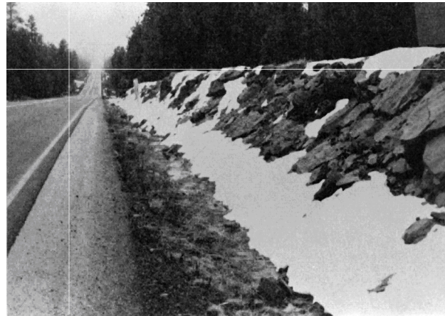
Figure 1160-6 Rural Roadside Hazard Rating of 6
