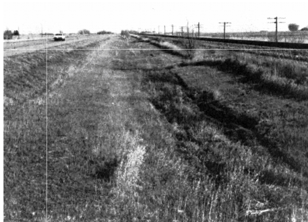
Figure 1160-2 Rural Roadside Hazard Rating of 2
