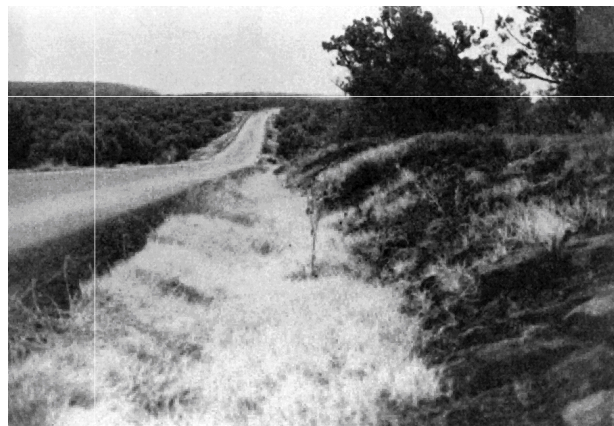
Figure 1160-3 Rural Roadside Hazard Rating of 3
